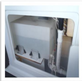
Potable Water Tank
